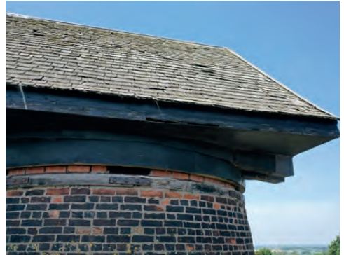
A drone survey showed the wooden roof shingles and facias in need of replacement and modern hard engineering bricks in use
